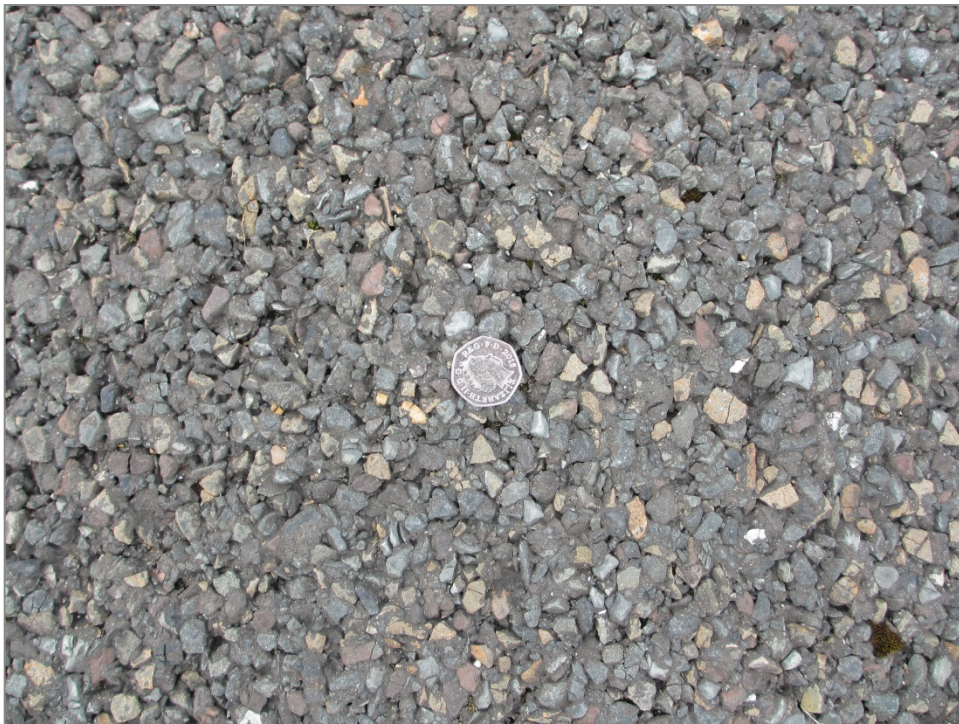
Figure: 9 Large aggregate used for wearing course may be impacting surface friction characteristics
