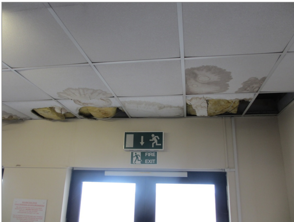
Figure 2: Evidence of water entering terminal building
